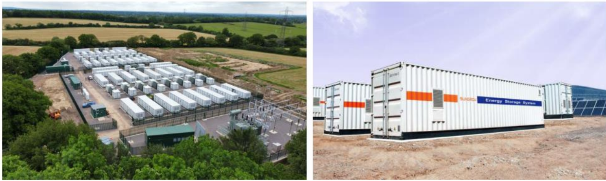
Figure 5 Example BESS storage area and 100MWH Storage Capacity
